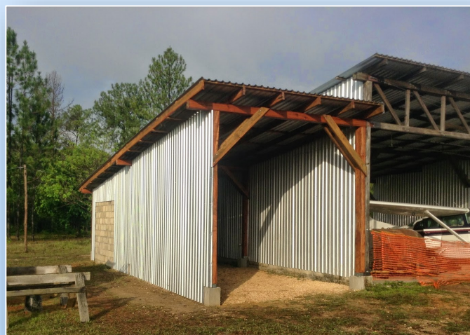
The new garage is ready and waiting to be filled with a new 4x4 utility truck for the mission base.
